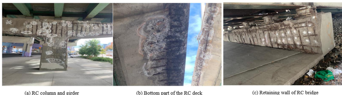
Figure 1. Corrosion of steel rebars in different members of the highway RC bridge in Canada.
