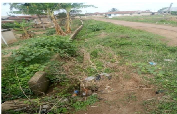
Figure 6. A typical drainage system in Ogbese showing blockage and structural failure.
