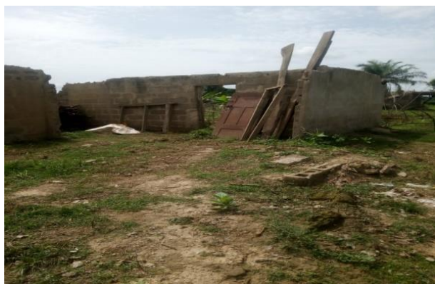
Figure 7. Structural collapse of a building resulting from flood action.
