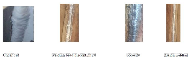
Figure 9. Various defect types observed at ABMI.
