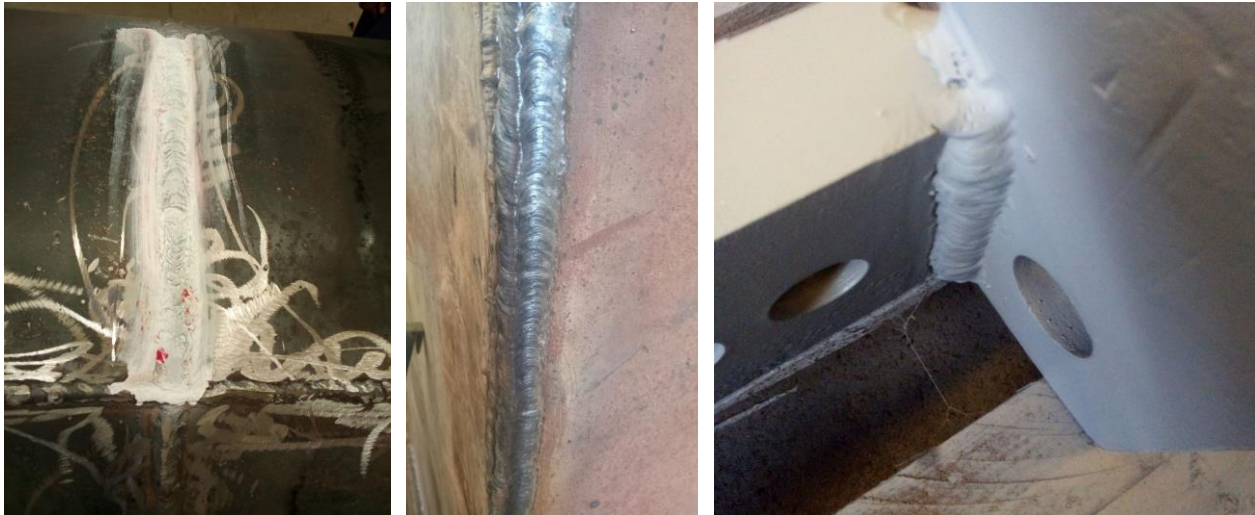
Figure 1. Welded products and their defects at ABMI.
