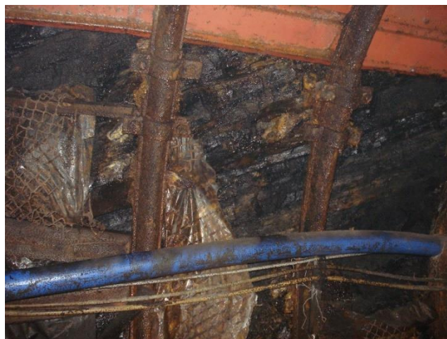
Figure 4. Isolation wall located towards the return air stream (no consequences of mechanical action).
